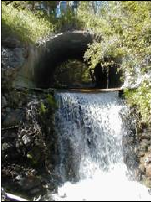
Figure 9-7. Photo of Impassable Fish Barrier at Forest Road 3413-110 (USFS 2007)
